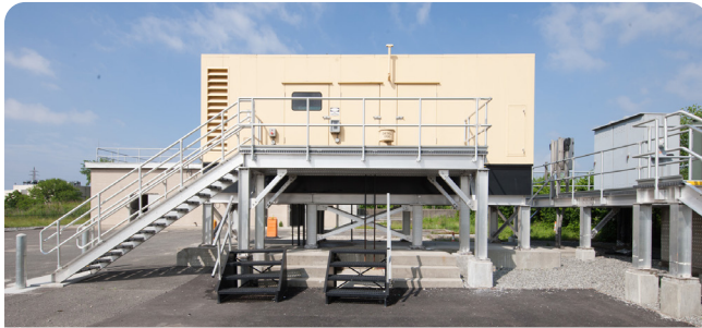
Flood Mitigation Measures at Four Sewage Pump Stations, Nassau County DPW.
