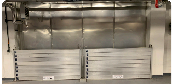
Flood Mitigation Measures included New Flood Water Gates at the Sludge Dewatering Facility, Superstorm Sandy Repair, Nassau County DPW.
