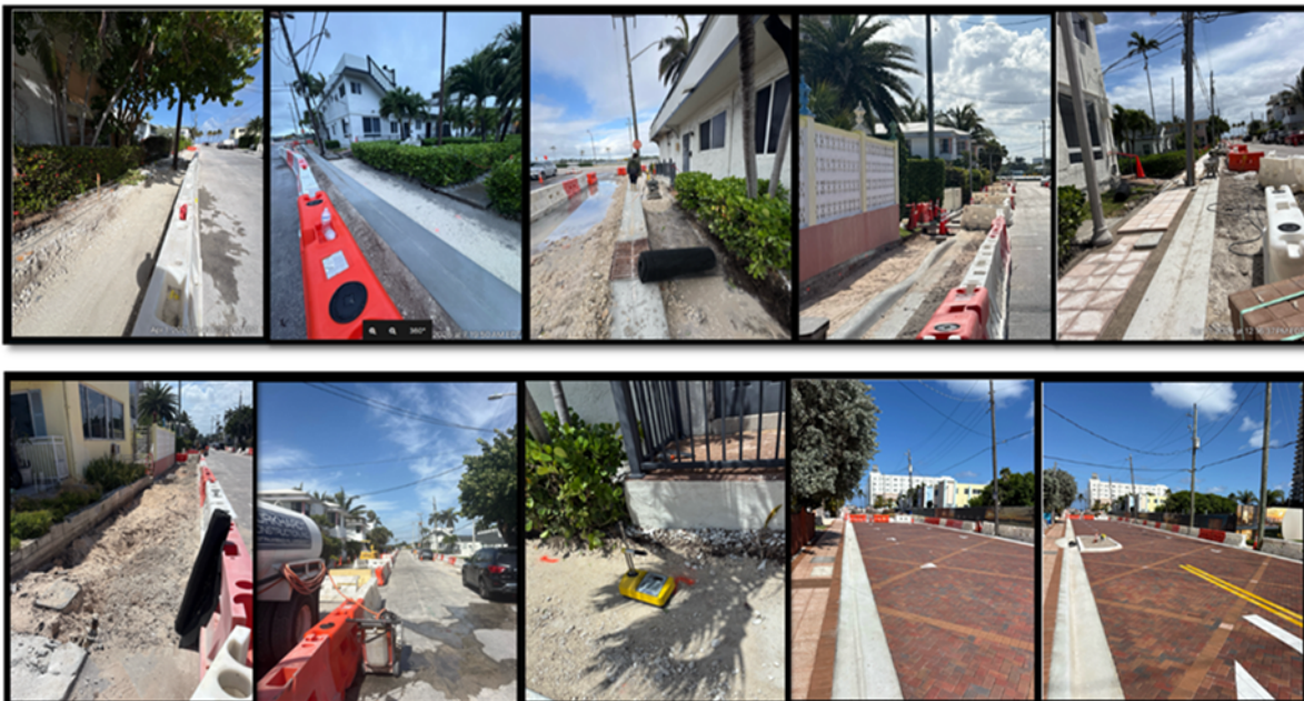
Demolition, filling, grading, compacting, and laying pavers on Georgia and Jackson Streets
