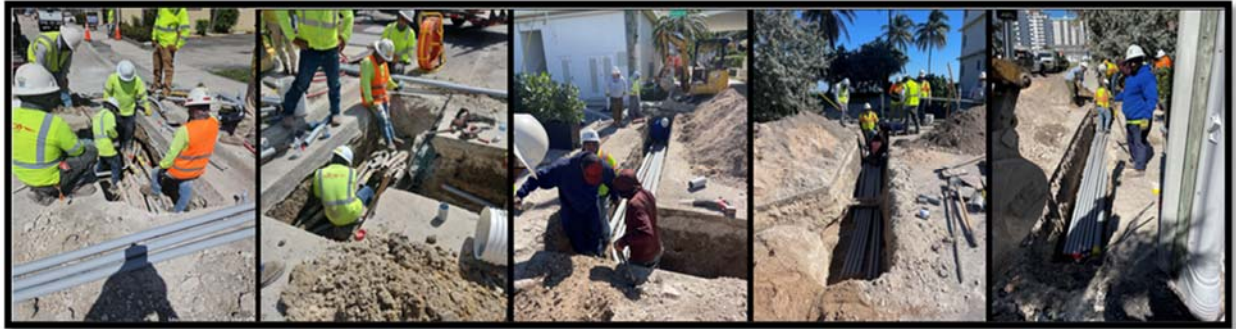
Open trench electrical and undergrounding at Georgia Street; conduit installation for FPL equipment "stub up"
