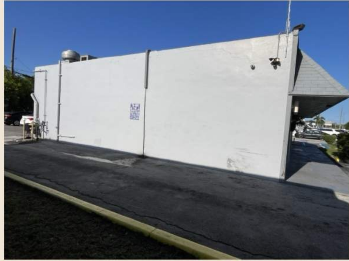
Left Side Existing Wall
