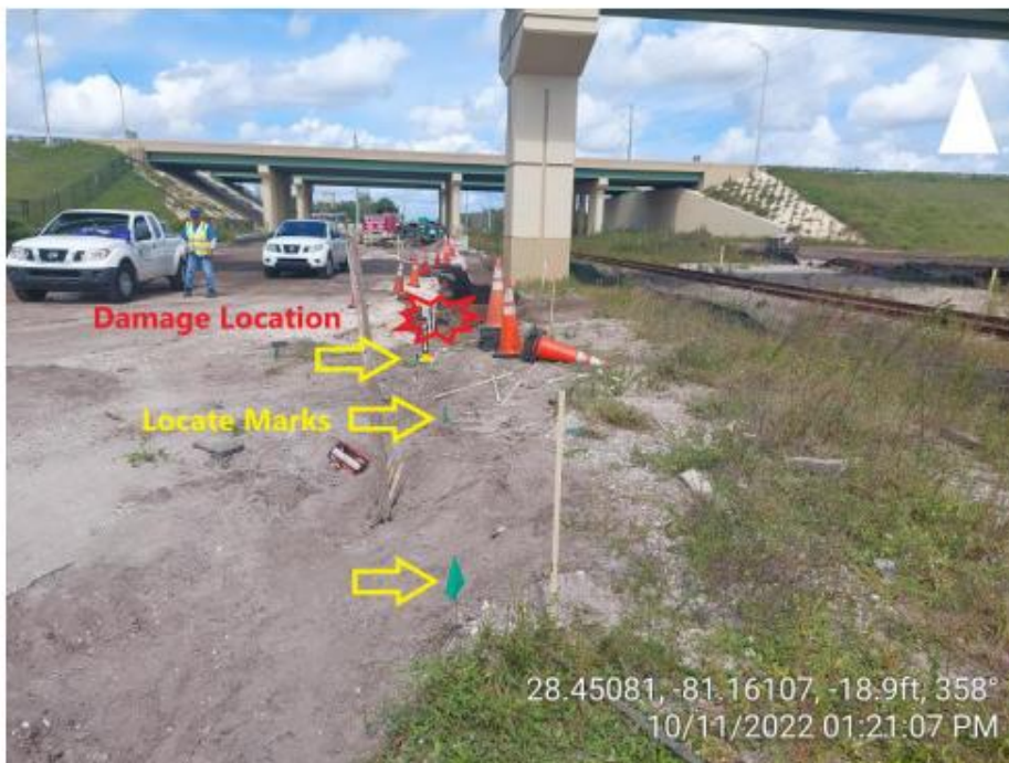
Pictures of the damage area taken 10/11/2022
