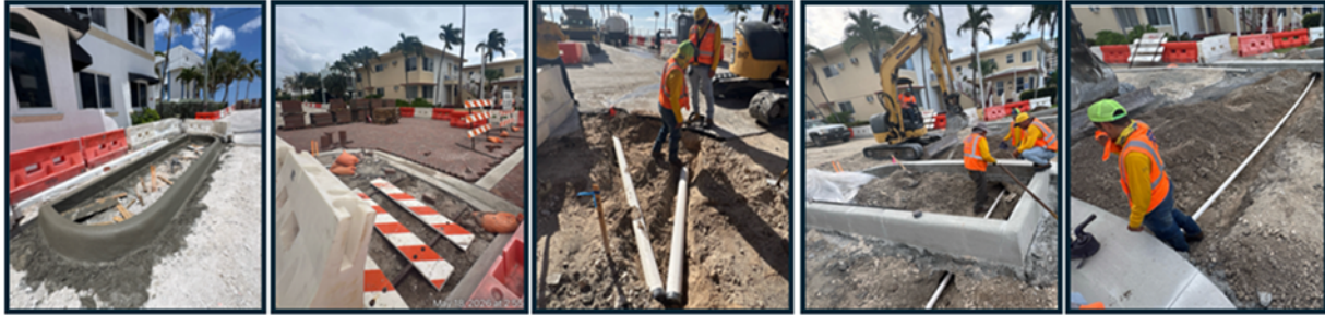
Jackson Street – transformer island layout and FPL equipment “stub up”
