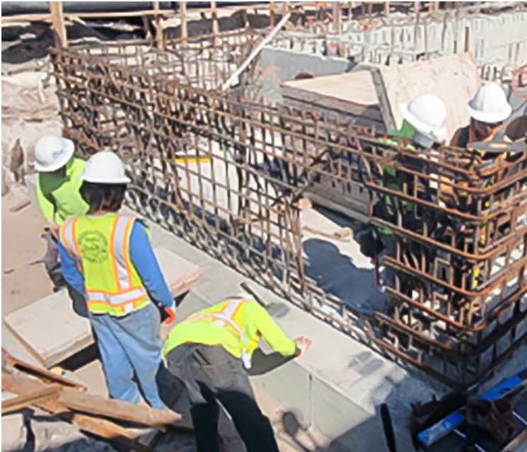
Interdisciplinary collaboration supports shared understanding, coordinated decision-making, and consistent project delivery across all phases.
