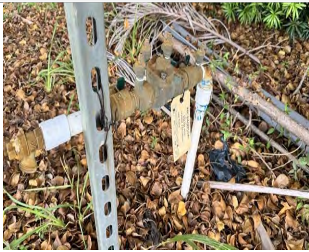
Utilities Mechanical Components
