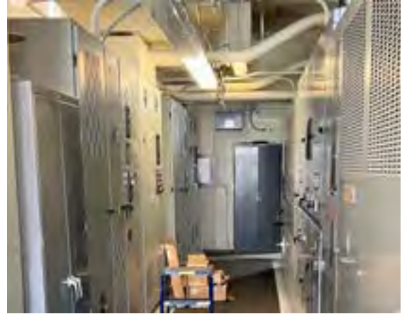
Space is limited for maintenance and operations with the existing equipment
