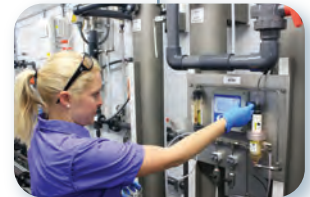
City of Hollywood SRWWTP Effluent Recharge Treatment Pilot Study $2.98 million
