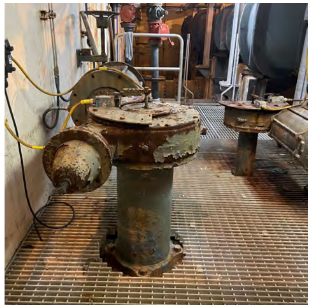
Corrosion and deteriorated coating observed.
