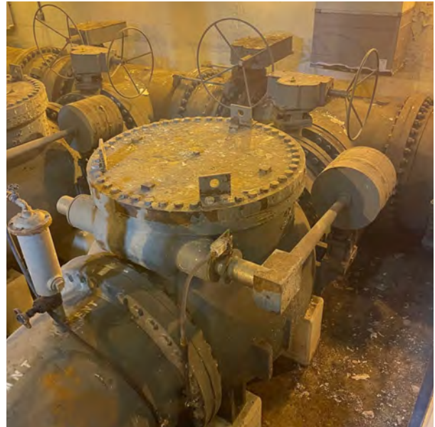
General view of the mechanical equipment for the pump discharge including a swing check valve.
