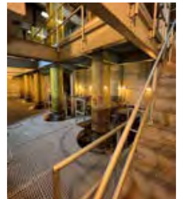
Extended shafts from existing IPS pumps, with motors mounted on the upper floor.
