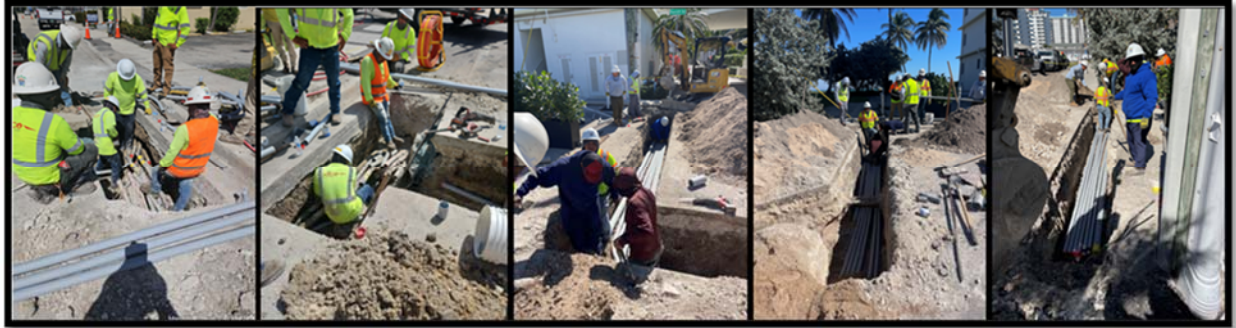
Open trench electrical and undergrounding at Georgia Street and Hyacinth Terrace; conduit installation for FPL equipment "stub up"
