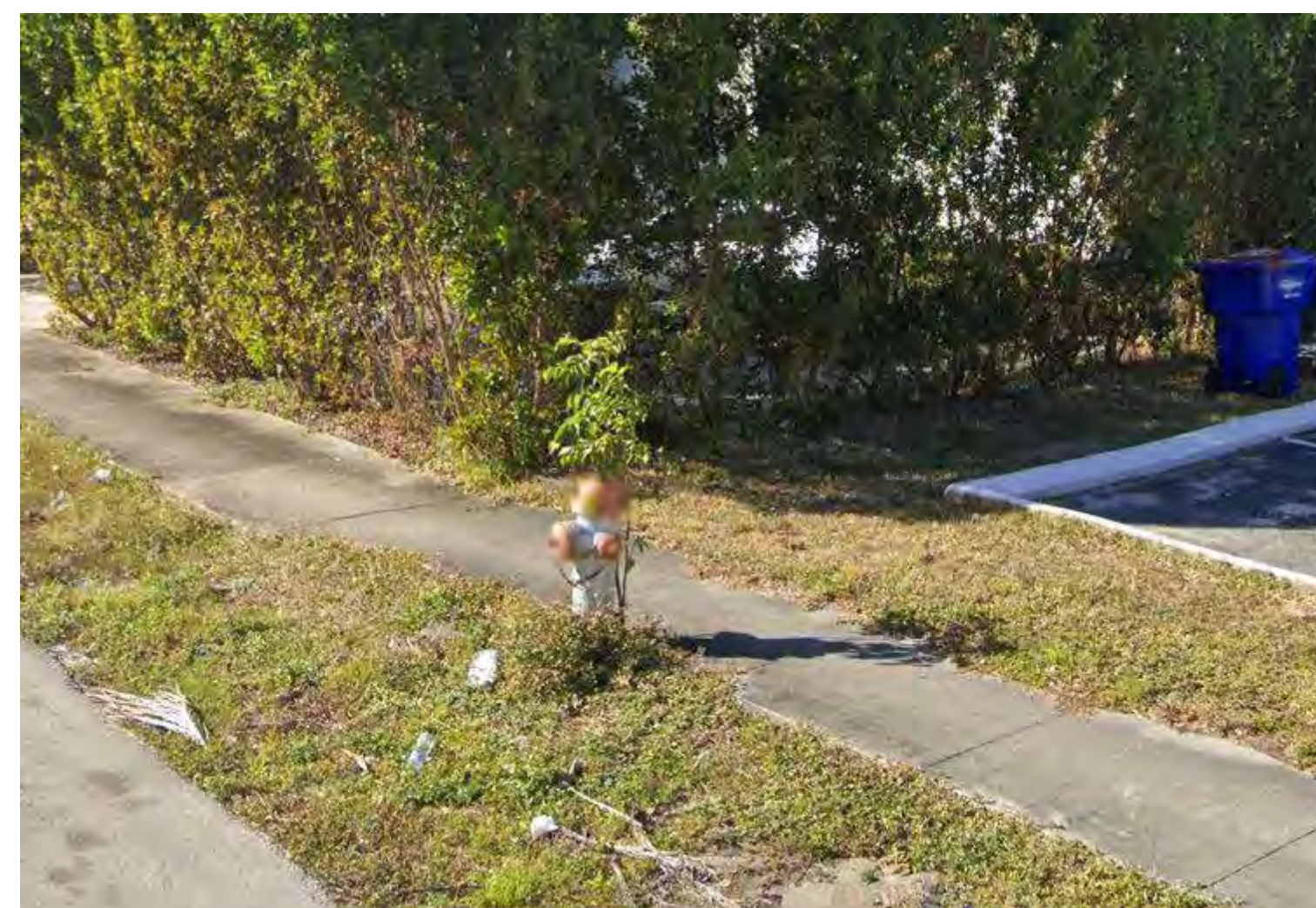
EXIST. FIRE HYDRANT 1
