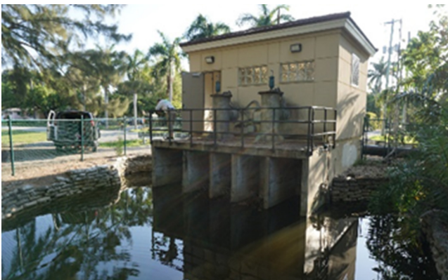
City of Hollywood Pump Station SW-06
