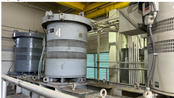
Photos of SRWWTP Influent Pump Station Pumps, Piping, and Control Panels
