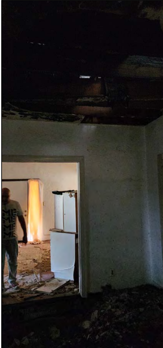
COMPLETE COLLAPSE OF FIRST FLOOR
