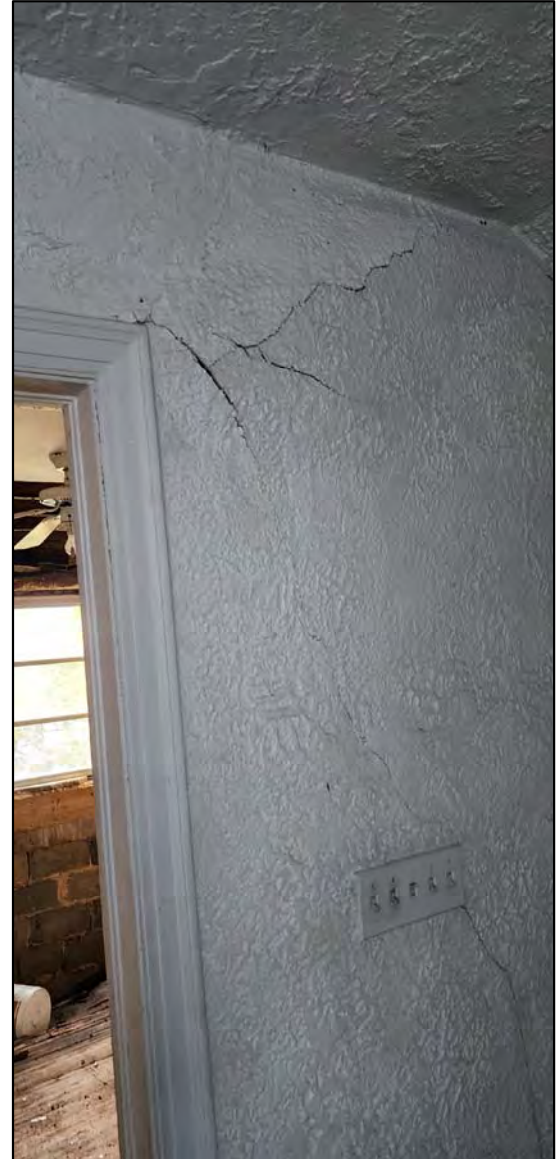
DIAGONAL CRACKS ABOVE THE DOOR
