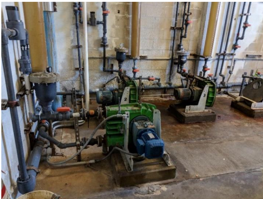
Figure 13. LS CL2/HEX Storage Chemical Feed Area LS CL2/HEX Storage Chemical Feed Area Pumps
