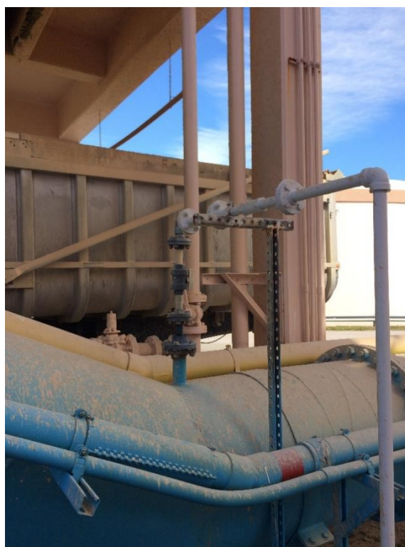
Figure 20. Existing Ammonia Injection Point
