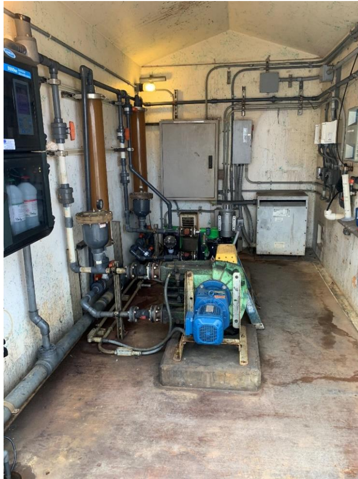
Figure 11. View of Odor Control Chlorination Building from Entrance
