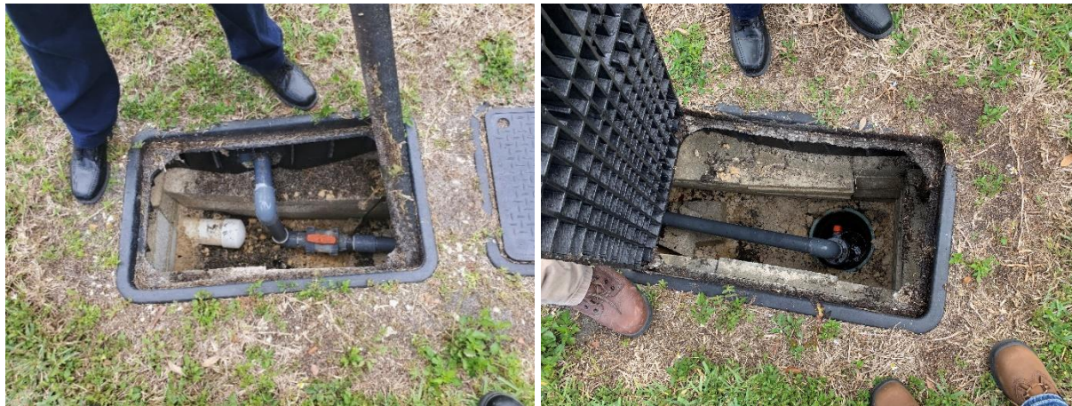
Figure 19. Chlorine Injection into Biscayne Raw Water to Lime Softener
