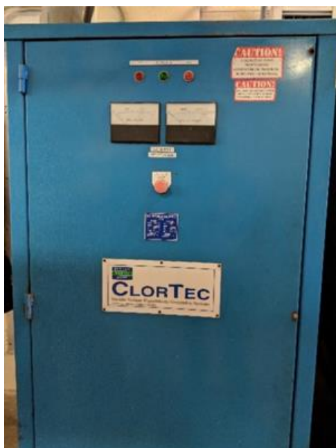
Figure 6. ChlorTec Rectifier Panel
