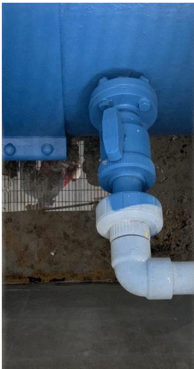
Figure 16. Injection Point at West Header
