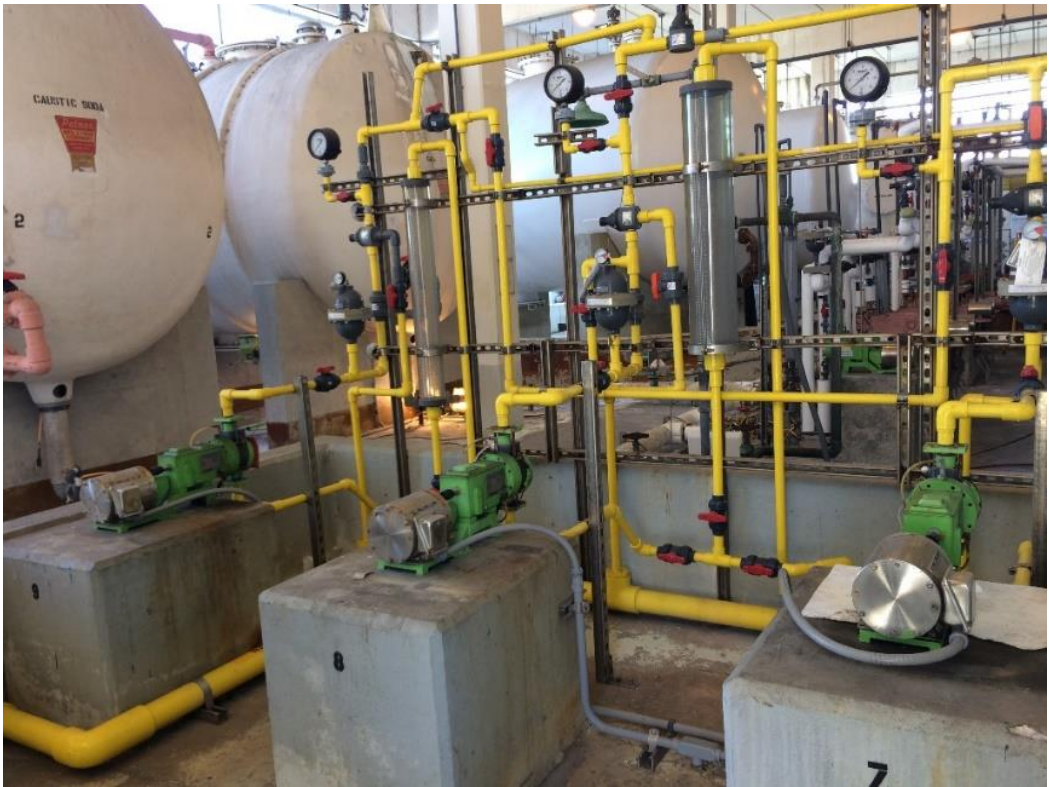
Figure 10. Membrane Building Chemical Storage Area Hypochlorite Metering Pumps
