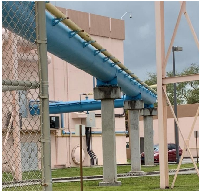
Figure 18. Post Filters 1 to 6
