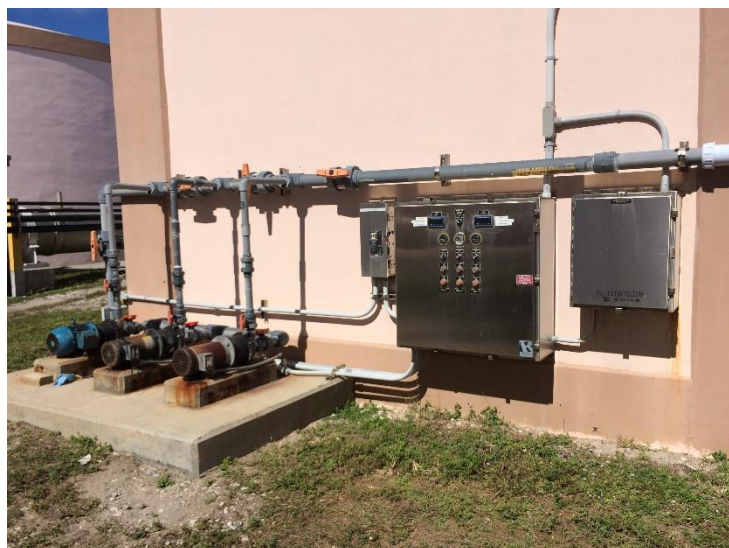
Figure 4. Transfer and Control Hardware Outside of the Chlorine Storage Building
