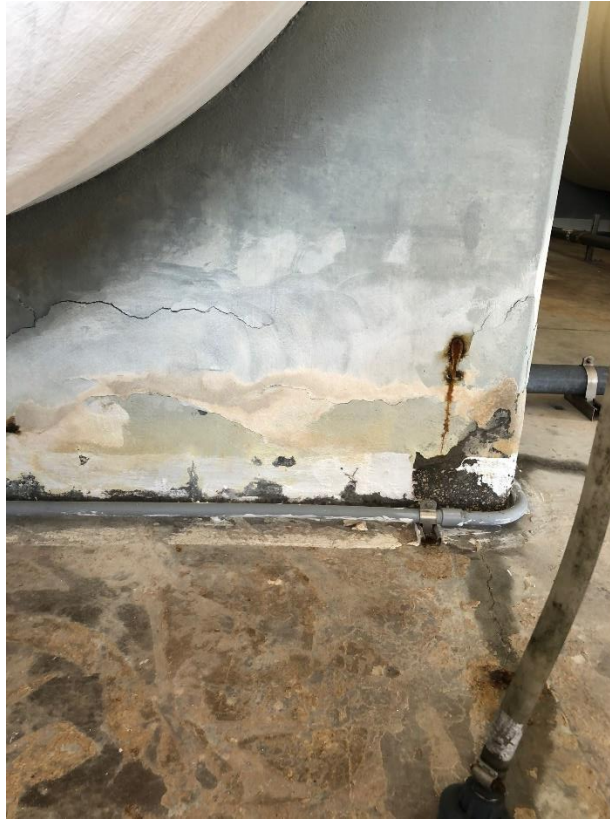
Figure 8. Concrete Saddle of Storage Tank in Chlorine Storage Building
