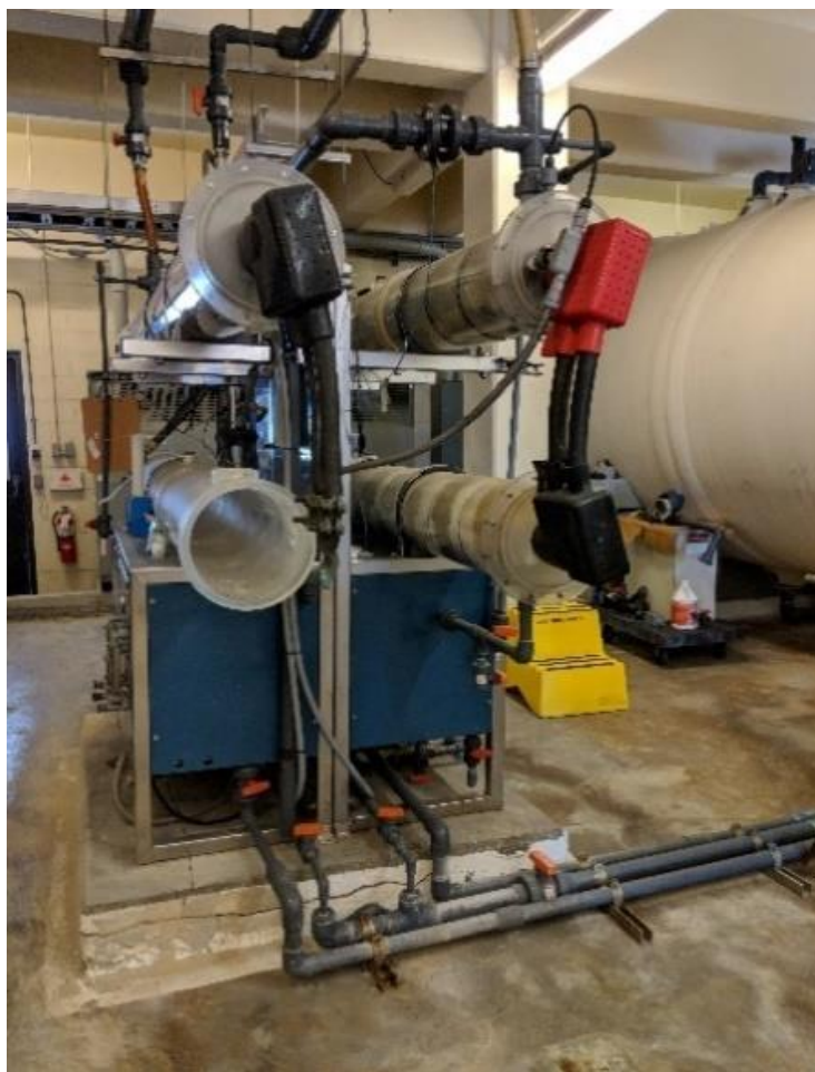
Figure 7. On-site Sodium Hypochlorite Generators
