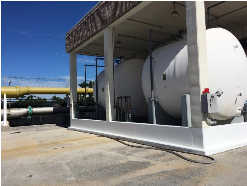
Figure 9. Two of Four Membrane Building Area Hypochlorite Tanks
