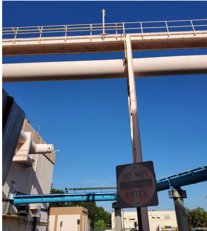
Figure 17. Lime-Softened Water from Spiractors 7 to 12 (Beige Pipe)
