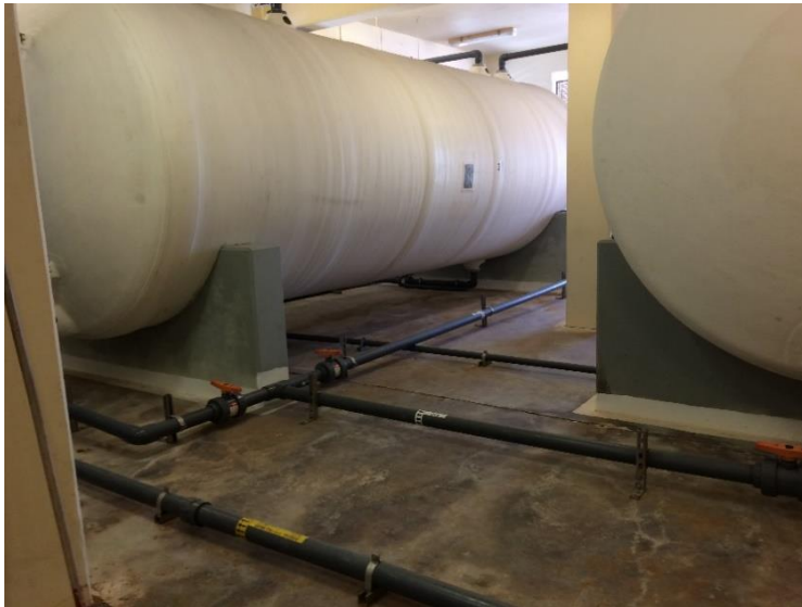
Figure 2. Chlorination Building Storage Tanks
