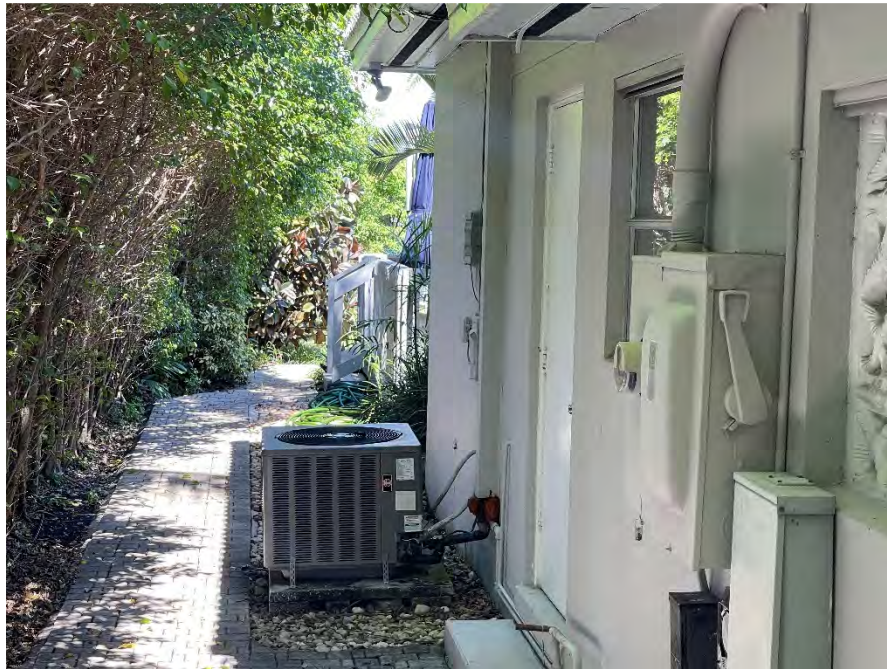
MEECH. EQUIP AT GRADE AND SERVICE EQUIP. VIEW
