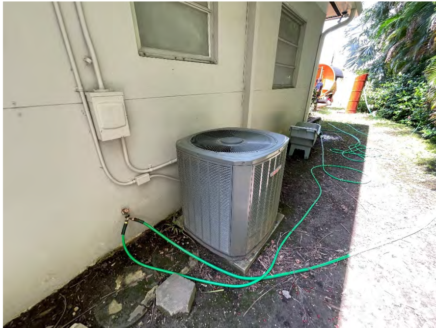
HVAC AT GRADE VIEW
