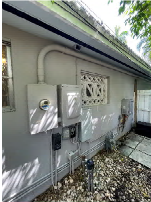
ELECTRIC SERVICE AT GARAGE AREA
