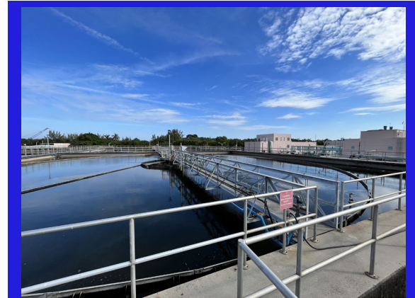
City of Hollywood's Southern Regional WWTP. The City intends to rehabilitate the existing clarifiers.
