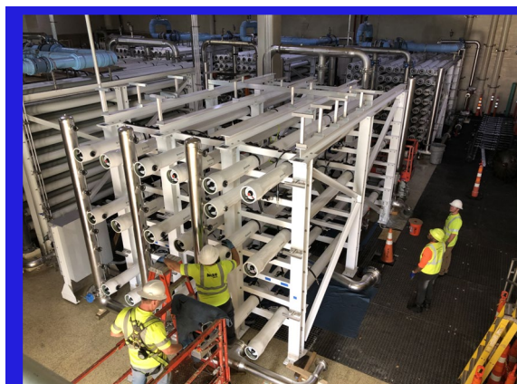
North Miami Beach NF & RO expansion. Jacobs brings market-leading membrane experience to the City of Hollywood, FL.
