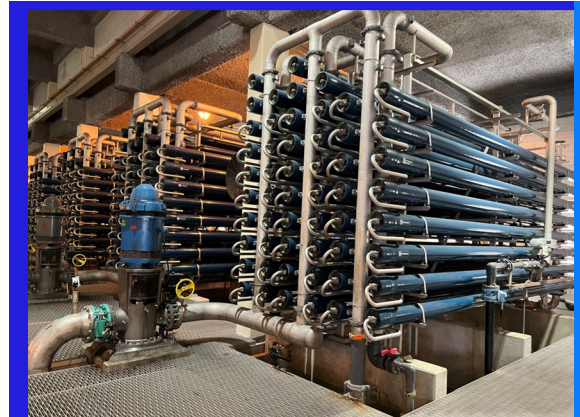
City of Hollywood WTP's existing membrane softening trains are arranged into a three-stage 32:16:6 configuration with seven element per pressure vessels and dedicated feed pumps.
