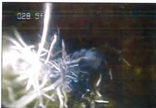
Roots in Sewer
