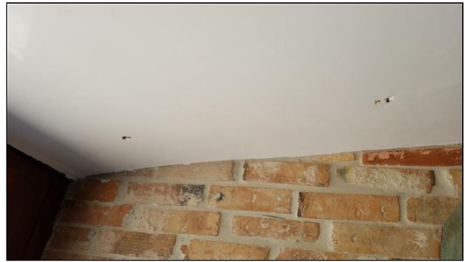
Ceiling damage due to termite
