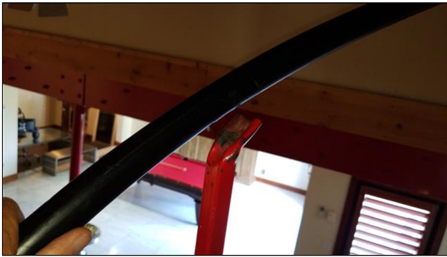
(3) Stairwell railing detached. $100
