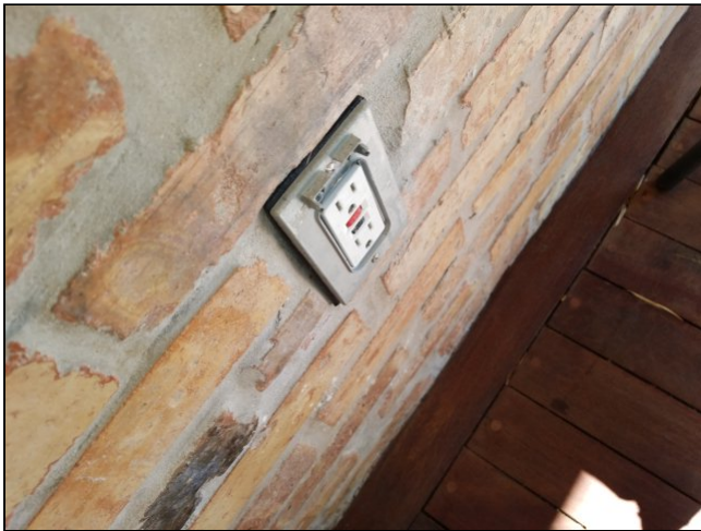
(33) No access to spa pool pump.
