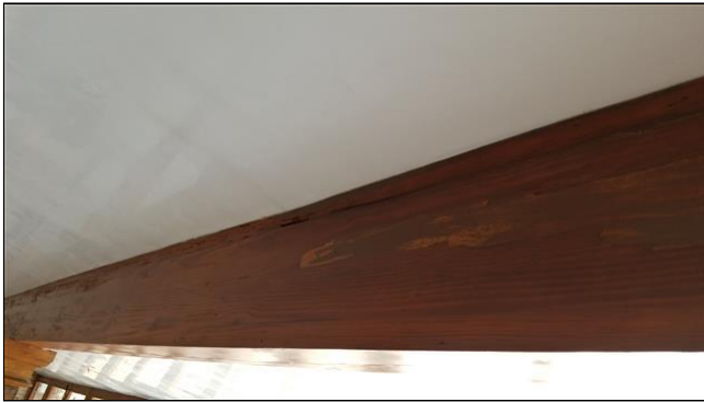
Termite damage to ceiling truss
