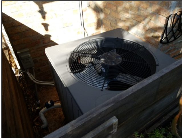
AC condenser unit
