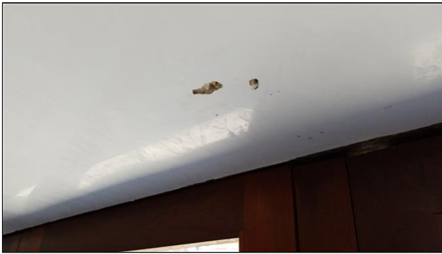
Ceiling damage due to termite
