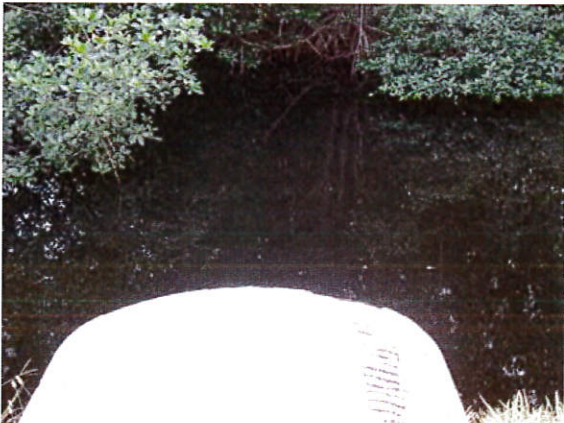
Example of public out-fall
