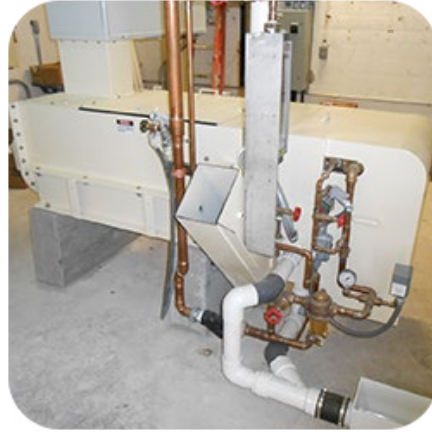
Public Water Supply District #2, Defiance MO
