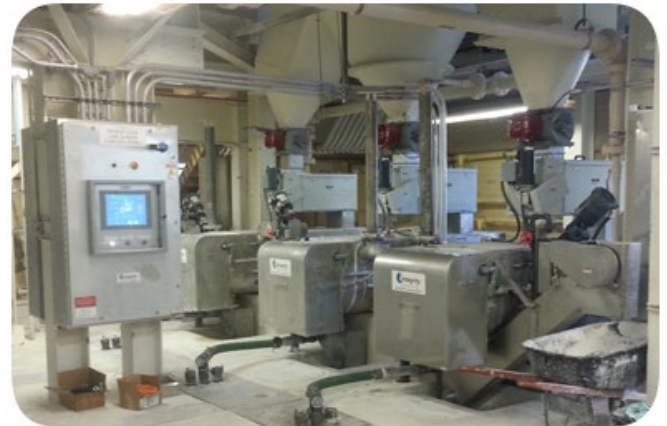
Davis WTP, Austin TX
