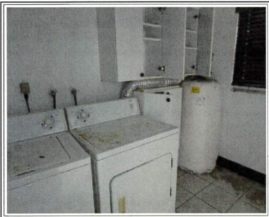
LAUNDRY / HOT WATER HEATER (WRAPPED)
