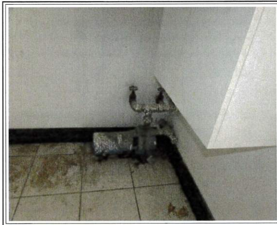
SPRINKLER WELL WATER PUMP
