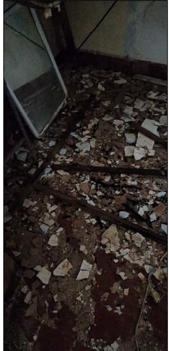
COLLAPSE OF ENTIRE FIRST FLOOR
