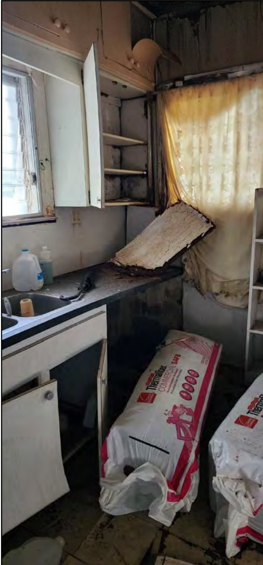
DAMAGED INTERIOR OF THE HOUSE (VERY POOR CONDITION)
