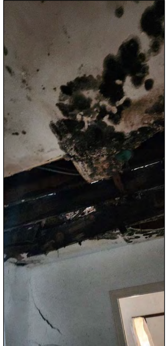
COLLAPSE OF INTERIOR OF FIRST FLOOR
