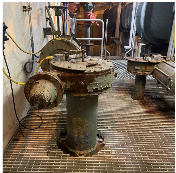
Corrosion and deteriorated coating observed.
