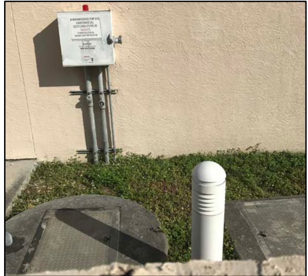
Photo 3-3. Private Lift Station E127-01
