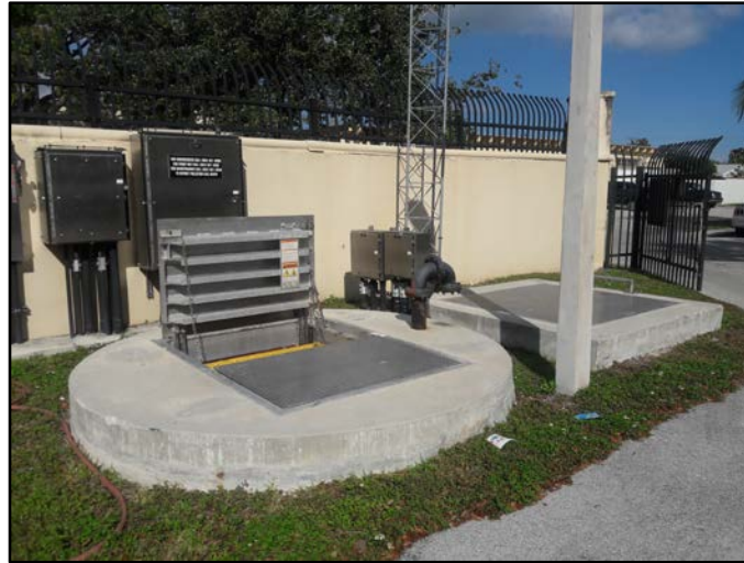
Photo 4-2. View of City Lift Station E-22 Wetwell
