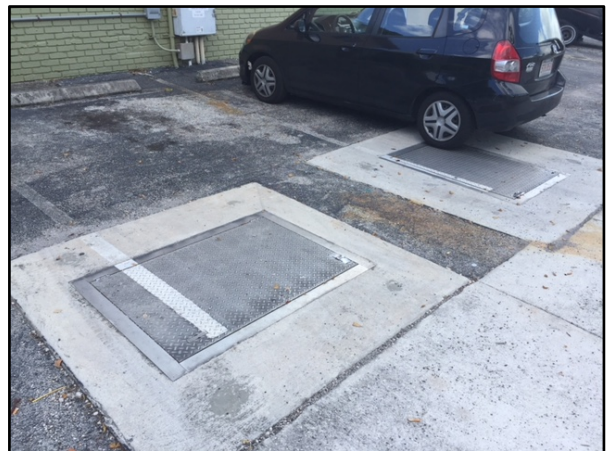
Photo 3-4. Private Lift Station E139-01
