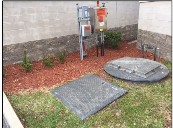
Photo 3-2. Private Lift Station E114-01
