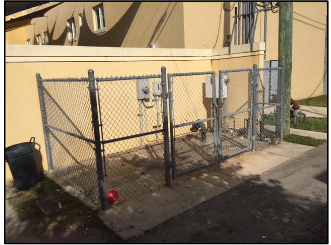
Photo 3-5. Private Lift Station E163-01
