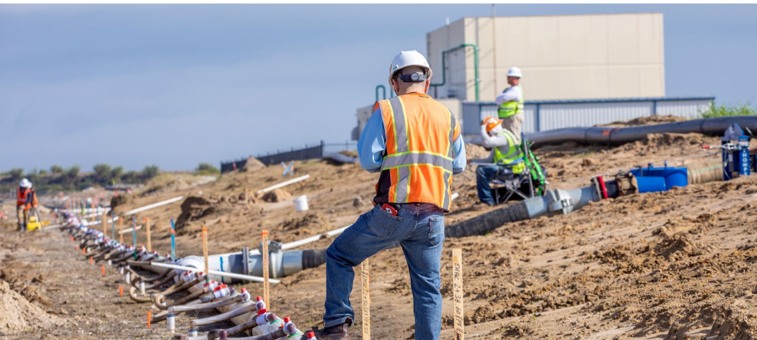
Pictured above: The HDR Team on-site at the Troup Indiantown Water Control District Pump Station Project (part of our C-44 Reservoir and STA contract with SFWMD).
