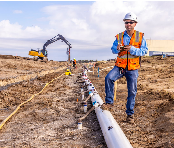
Pictured above: The HDR Team on-site at the Troup Indiantown Water Control District Pump Station Project (part of our C-44 Reservoir and STA contract with SFWMD).
