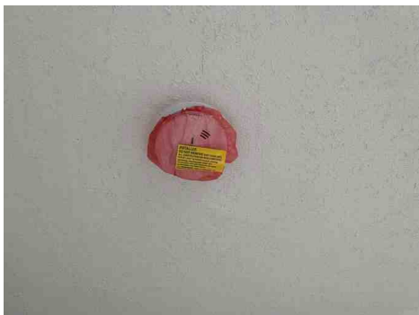
CO - Smoke Detector
