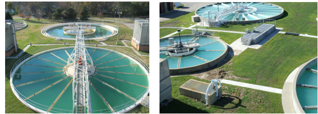
Lime softening basins operating in conjunction with membrane treatment at Olathe, KS, 37-mgd WTP.
