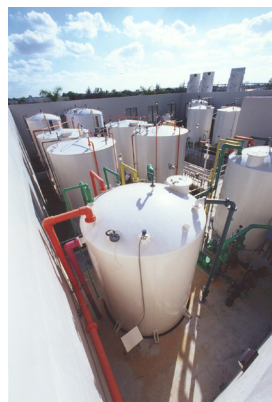
Sulfuric acid and scale inhibitor have been industry standard chemicals for pretreatment.
