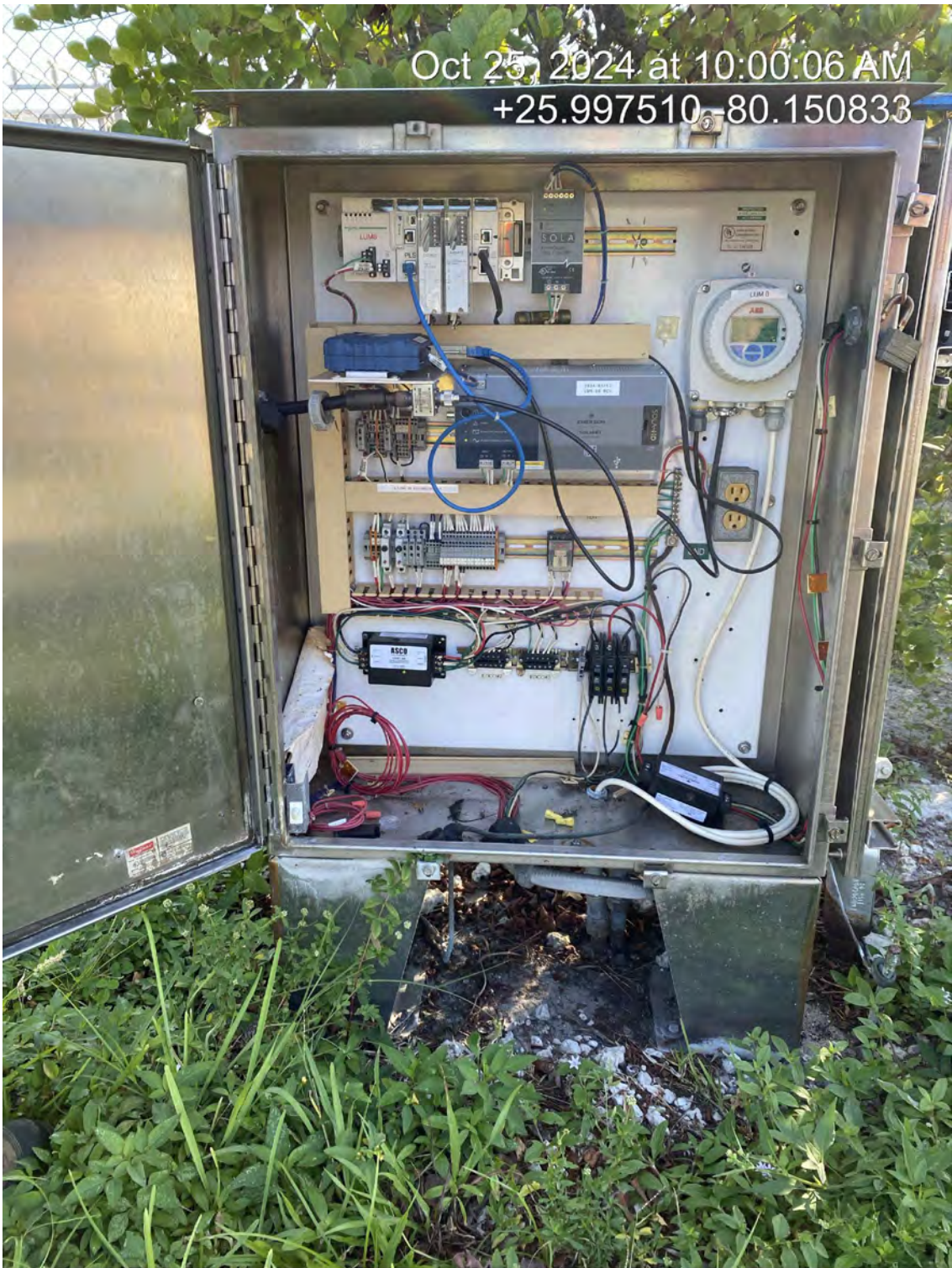
LUM 08 ELECTRICAL PANEL TO BE RAISED 30" ABOVE THE GROUND
