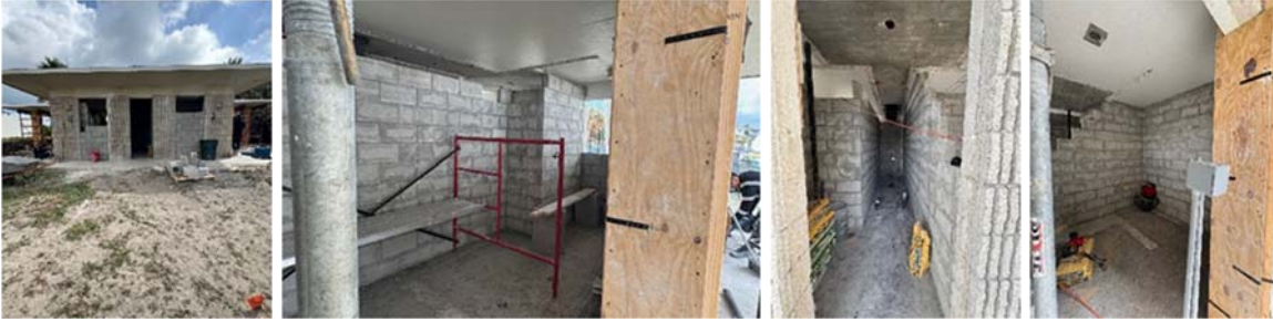
From Left to Right: 1. Filling the existing door openings, 2. Block partition installation (int. view from storage room) 3. Block partition installation (int. view from plumb. chase), 4. Block partition installation (int. view from bathroom)
