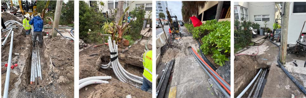
Undergrounding and electrical infrastructure installation, private property conduit runs, fire hydrant relocation
