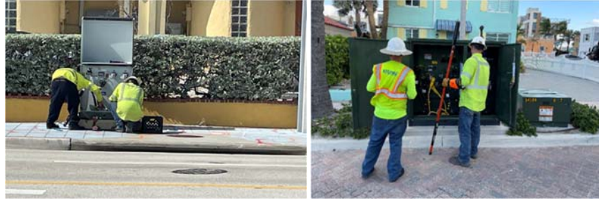
FPL energizing transformers and switching activities
