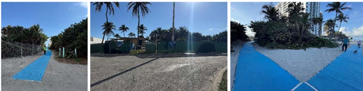
From Left to Right: 1. Site fencing installation, 2. Site fencing & signage installation completed. 3. Public Works & Beach Maintenance installed Access Mats for pedestrian access during construction.
