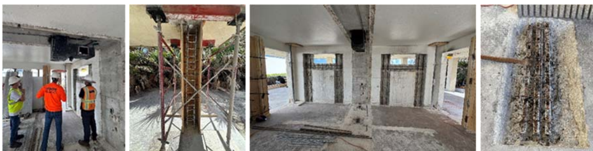
From Left to Right: 1. On-site meeting for structural remediation efforts, 2. Forming of existing column to be repaired and repoured, 3. Interior view of east wall to be reinforced, 4. Condition of slab to be restored.
