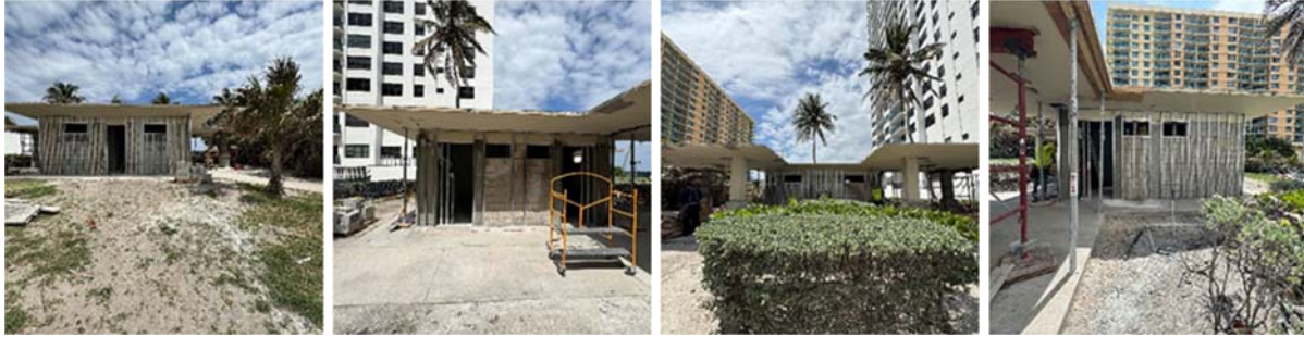
From Left to Right: West elevation; south elevation; east elevation; north elevation framing.
