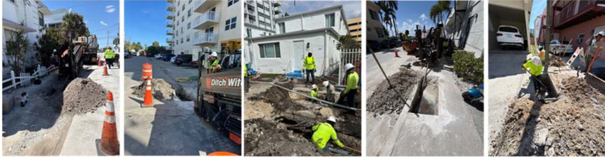
Undergrounding and electrical infrastructure installation, private property conduit runs, fire hydrant relocation
