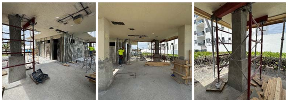
From Left to Right: Column A2 repair complete; Columns C3 & D3 Prep & Pour; Column D2 repair complete.
