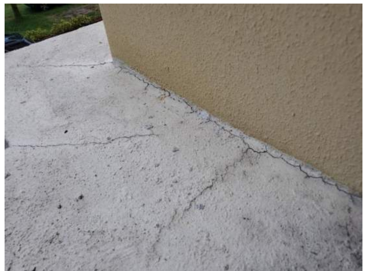
Figure 7. EIFS Cracking at Van Buren Garage
