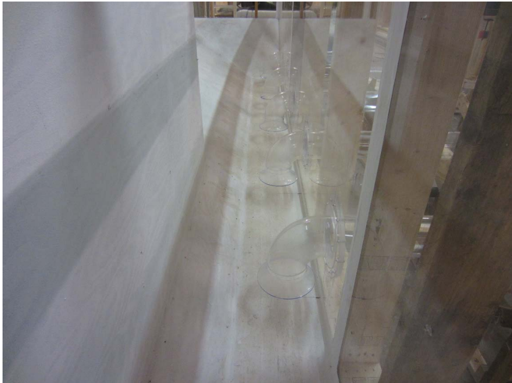
Photo 2 Similar Wet Well with Multiple Pump Suctions
