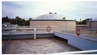
JEA Arlington East WRF BNR Upgrade 2011 FICE Engineering Excellence Award
