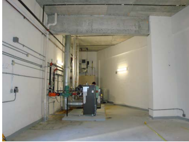
Raised floor slab and evidence of standing water
