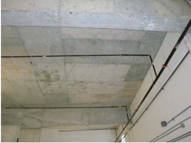
Fire Suppression System to be Relocated
