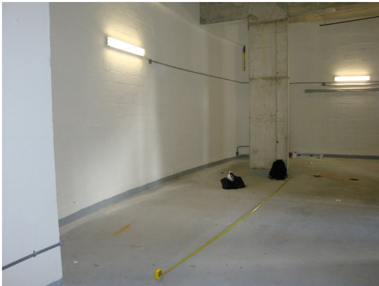
Column interference in Equipment Room Location
