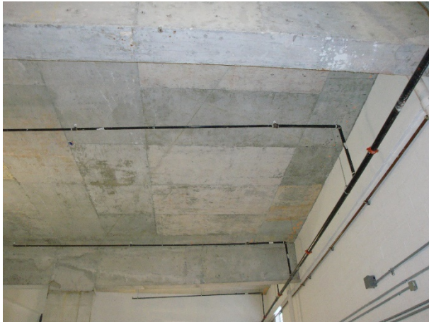
Fire Suppression System to be Relocated
