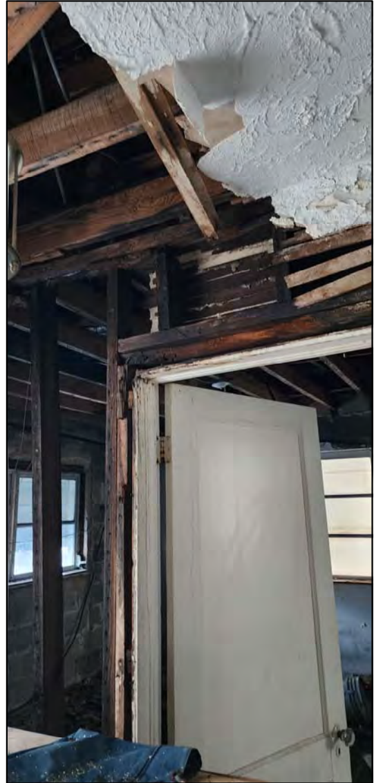
DAMAGED INTERIOR FRAMING
