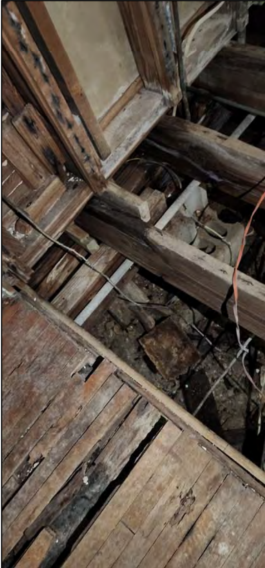
COLLAPSE OF THE FIRST FLOOR AND EXPOSED DETERIORATED FLOOR JOISTS AND WOOD STUDS
