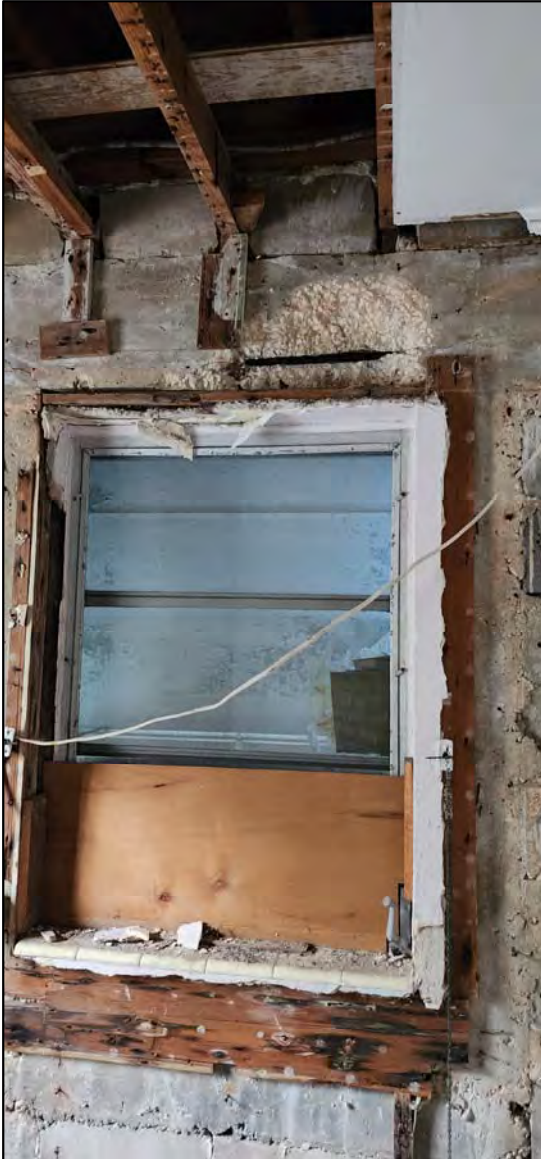
DETERIORATED WINDOW FRAME AND EXPOSED RUSTED REINFORCING IN CONCRETE BEAM
