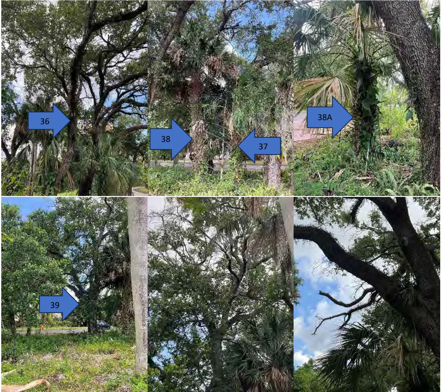
Live Oaks ( Quercus virginiana ) Tree #'s 36 & 39, and Sabal Palms ( Sabal palmetto ) Tree #'s 37, 38 & 38A, facing west. Note poor structure, canopy crowding, large diameter deadwood for Tree # 36, and Poor structure, canopy crowding, large diameter deadwood, canopy dieback for Tree # 39.
