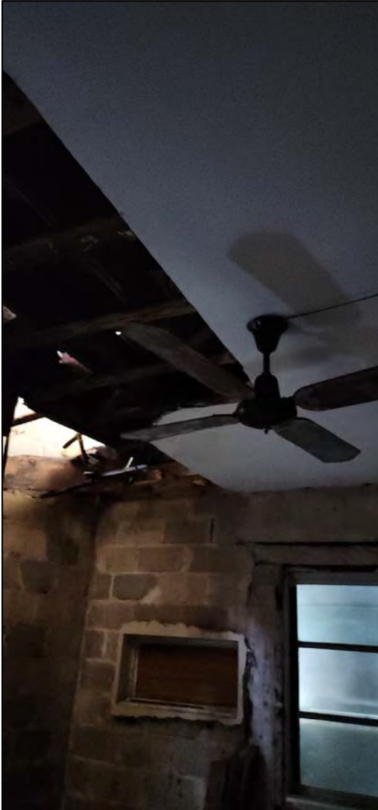
DAMAGED SECOND FLOOR
