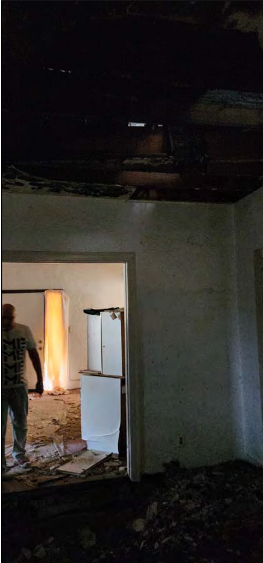
COMPLETE COLLAPSE OF FIRST FLOOR
