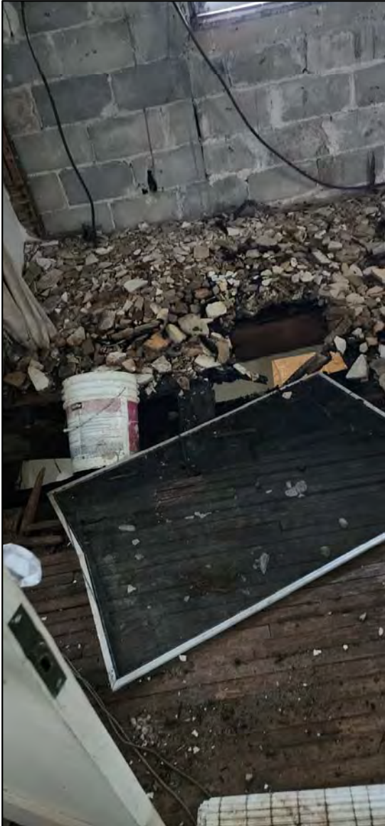
COLLAPSE OF FIRST FLOOR
