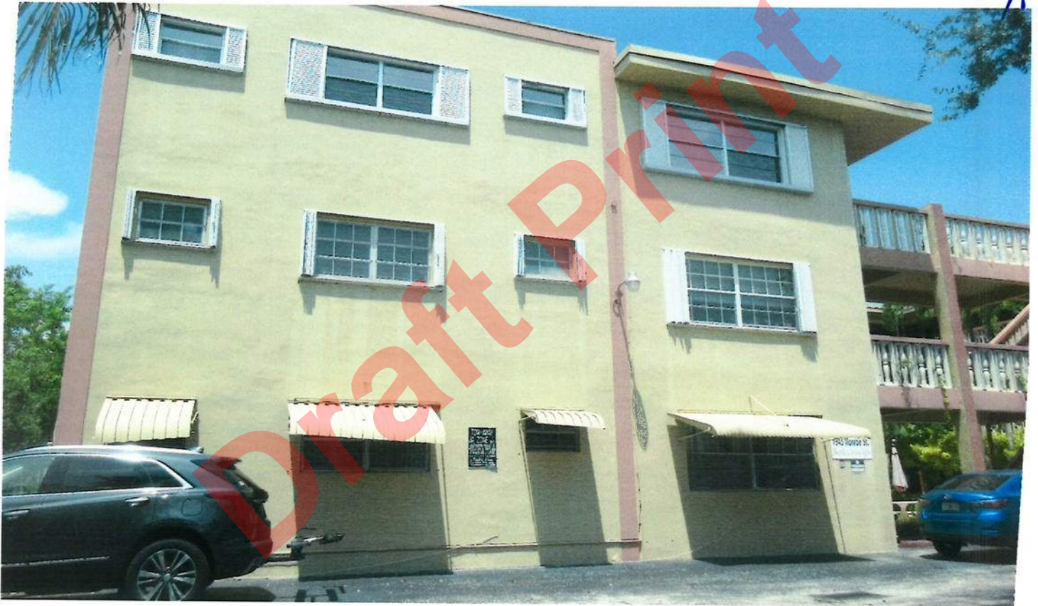
Outer tops and sides of clam shell awnings are to be repainted. A good amount of extra labor time is expended in order to properly cut in paint around the outer and inner portions of hurricane shutters.
