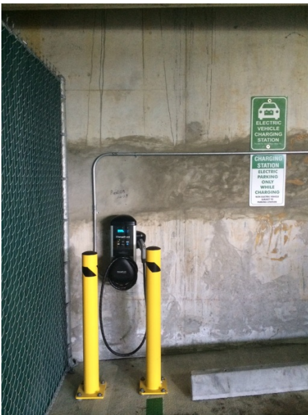
Figure 7: Electric Charging Station at the Radius Garage
