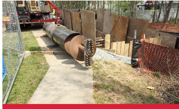
Figure C.4-4. Riedel Road Water Main. Gannett Fleming provided CM/I services, survey, E&SC compliance, and specialized testing for the installation of 3,200 LF of new 16-inch water main.
