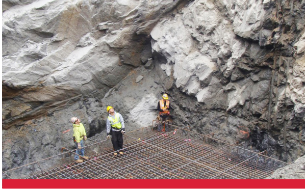
Figure C.4-8. Chester-Ridley Creek Sewer Reroute. The force main alignment presented challenges, including crossings under I-95, railway crossings, and numerous utility conflicts.
