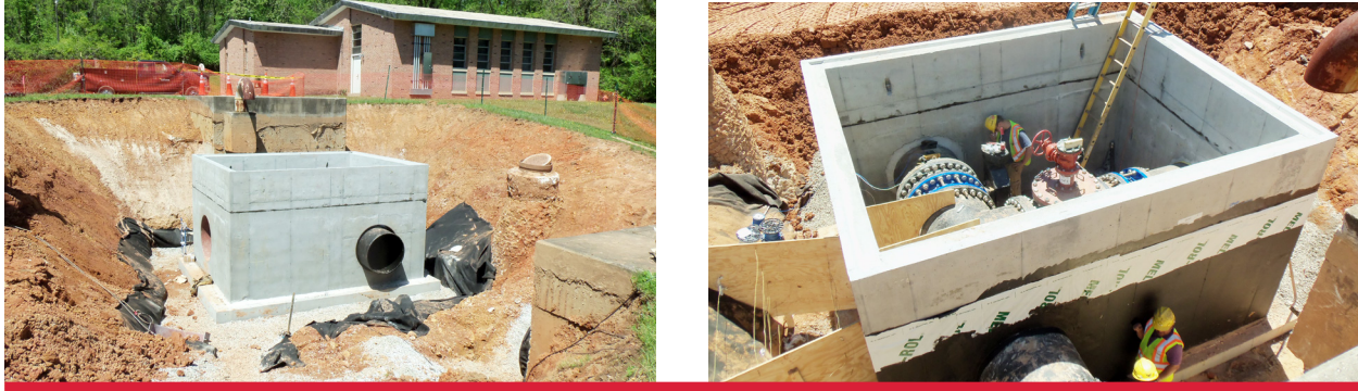
Figure C.4-6. Catonsville Pump Station Upgrades. On Gannett Fleming’s recommendation, the County split the project into two separate construction contracts, which improved quality, reduced contract costs, and assisted the County with funding.
