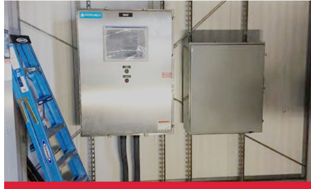
Figure C.4-10: Pump Station Improvements. As part of the design, Gannett Fleming made sure all electrical equipment was elevated above the 100-year flood plain.
