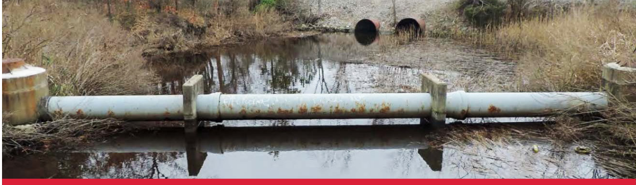
Figure C.4-5. Ferebee and Park Avenue Pump Station Pipeline Design. The existing pipeline between the two stations consists of approximately 7,000 LF of 12-inch force main and 24- and 18-inch gravity sewer. Gannett Fleming’s updated design is expected to include approximately 2,600 LF of 12-inch force main, and 6,600 LF of 30-inch gravity main to connect the new pumping stations.
