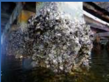
Oyster-Encrusted Bridge Piling
