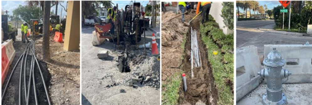
Undergrounding and electrical infrastructure installation, private property conduit runs, fire hydrant relocation
