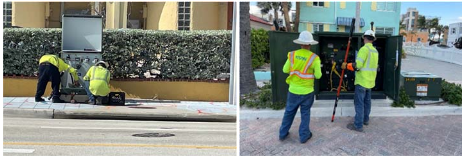
FPL energizing transformers and switching activities
