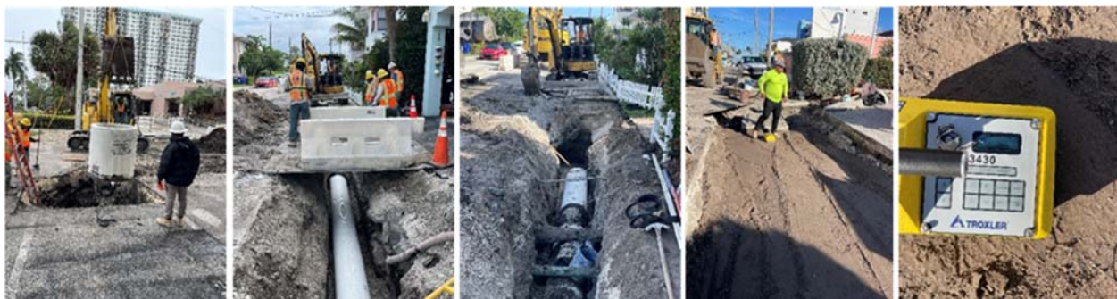
Drainage structure and pipe installation, setting up structure and pipe, and compaction (Harrison and Van Buren Streets, Bouganvilla Terrace)
