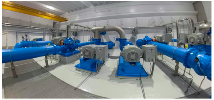
High-Service Pumping Station Completed in 2019
