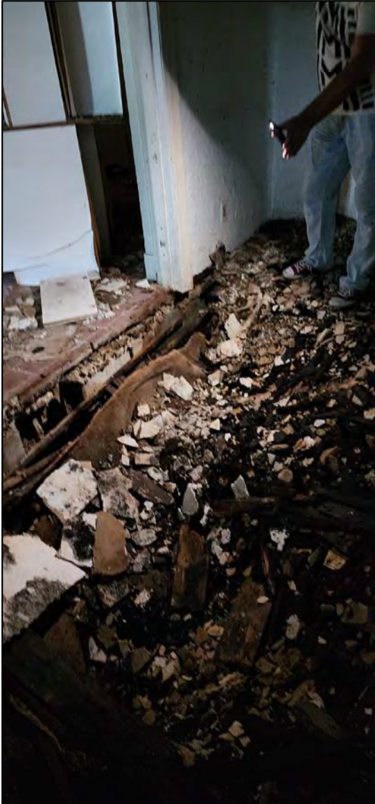
COLLAPSE OF FIRST FLOOR AND DETERIORATED MEMBERS
