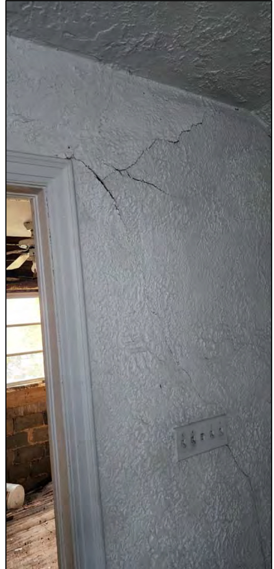
DIAGONAL CRACKS ABOVE THE DOOR
