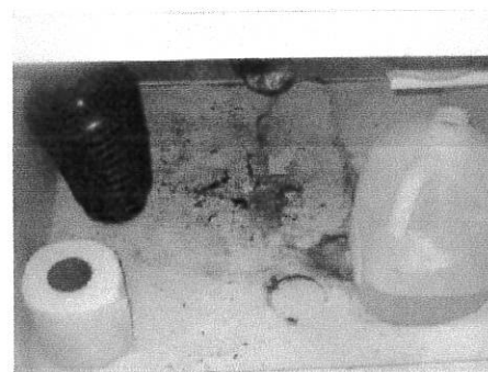
Photo #19 DAMAGED VANITY DUE TO DRAIN LEAK.
