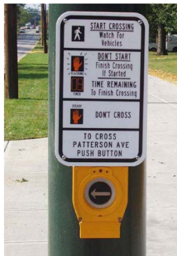
Pedestrian Activated Signals
