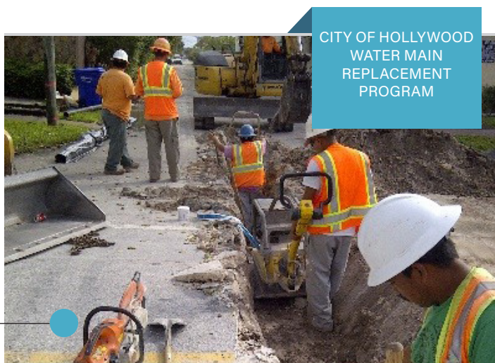
TETRA TECH HAS DESIGNED OVER 50 MILES OF WATER MAIN REPLACEMENT FOR THE CITY'S WATER MAIN REPLACEMENT PROGRAM
