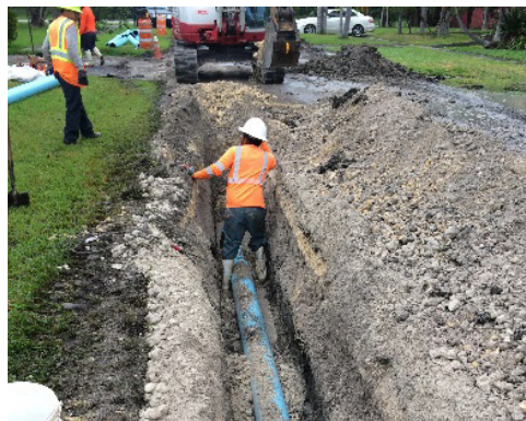
TETRA TECH HAS ASSISTED WITH CONSTRUCTION ADMINISTRATION OF THE WATER MAIN REPLACEMENT PROGRAM
